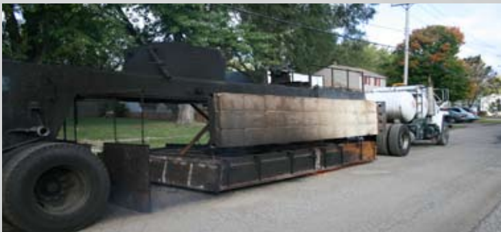
The first of two machines that pre-heats the existing paving material. Note the extensive cracking and wear of this residential street.
