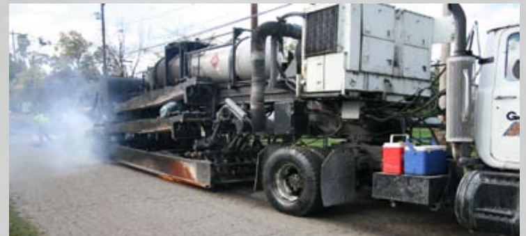
The second machine raises the temperature of the asphalt even higher, before applying an oil/polymer mixture to rejuvenate the asphalt.
