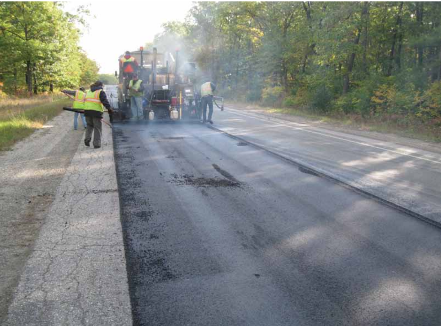
After Gallagher finished its preservation work, Rieth-Riley, Traverse City, MI, placed 4,000 to 5,000 tons of a low (traffic) volume Superpave ultra thin mix.
