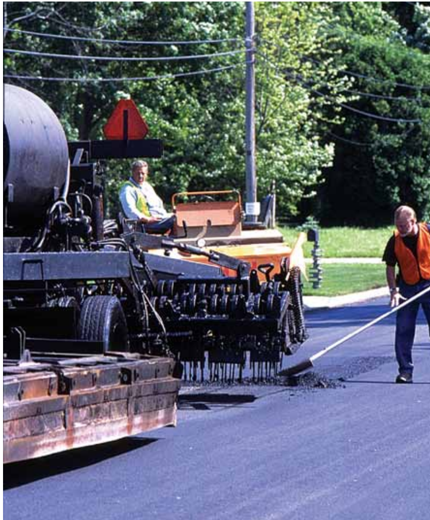
While Gallagher has offered Hot-in-Place recycling for a long time, it's only been in the past three or four years that customers have begun to realize the cost and other benefits this method can provide.
